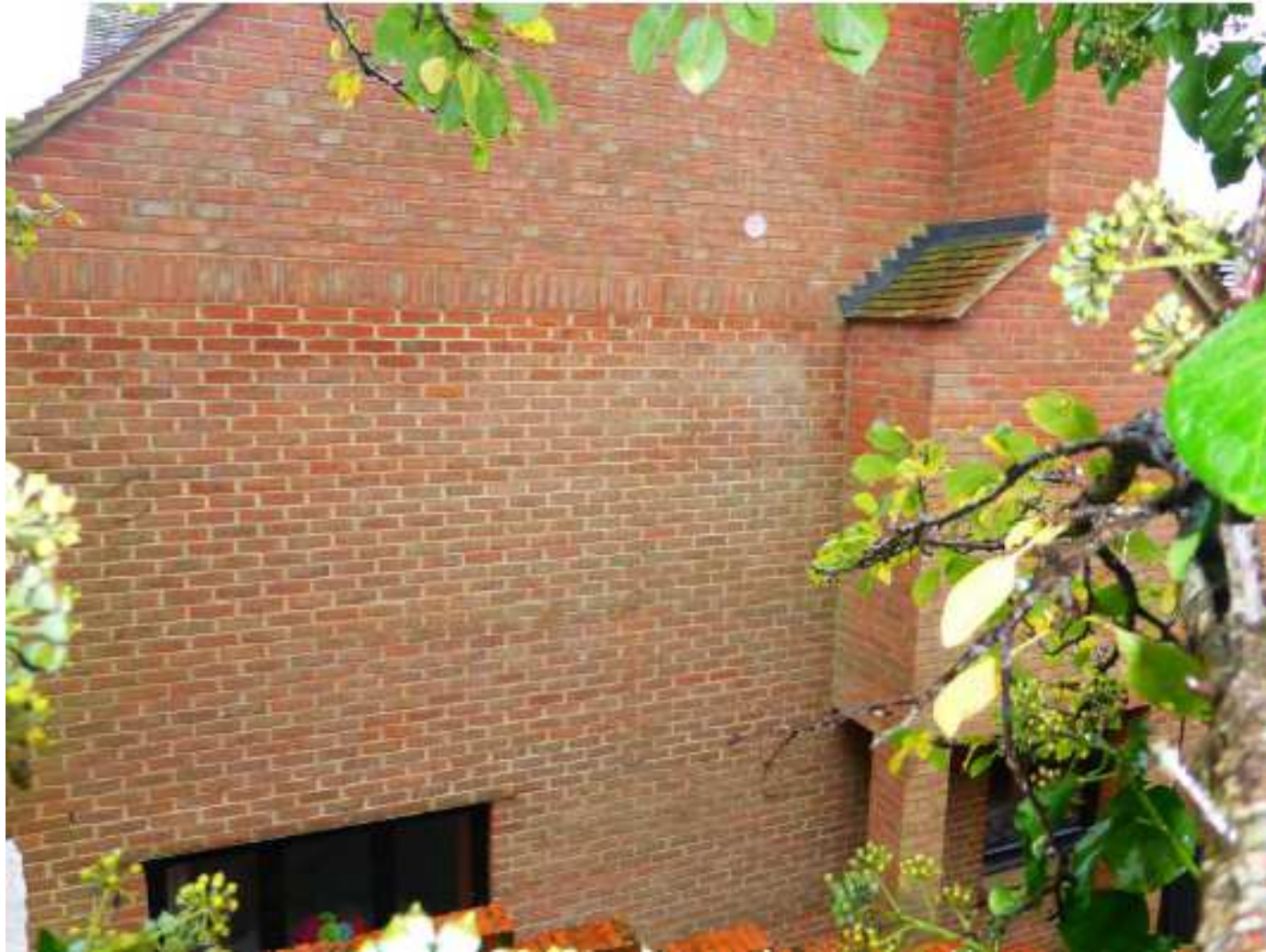
Side elevation of neighbouring dwelling (Mountain Ash) that this proposal is adjacent to.
